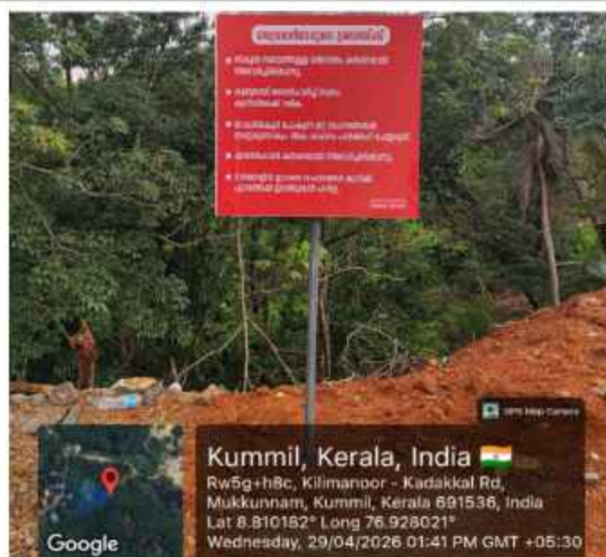
Figure 1: Caution board for truck drivers
